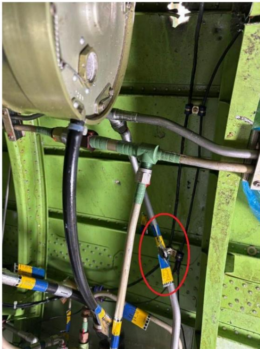
Fig. 15. Hydraulic system 3 – damaged tube
