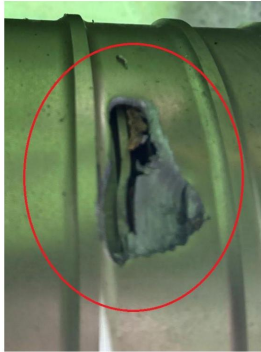
Fig. 19. Hydraulic system 3 – detailed view of the damaged tank
